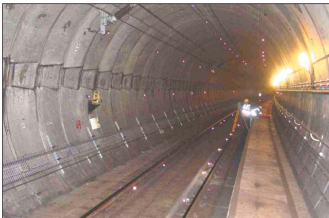
Obr. 12 Monitoring tunelu trati Heathrow Express (automatický teodolit a terče) Fig. 12 Monitoring of Heathrow Express tunnel (robotic theodolite and targets)
